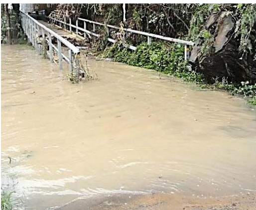
Photo: The Merri shared path is underwater just downstream of Bell Street Coburg, a few hours after the flood.
